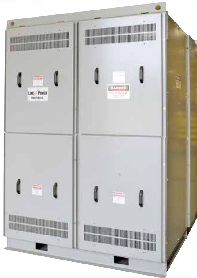
Indoor 5 kV Generator Switchgear For Water Shed Control
