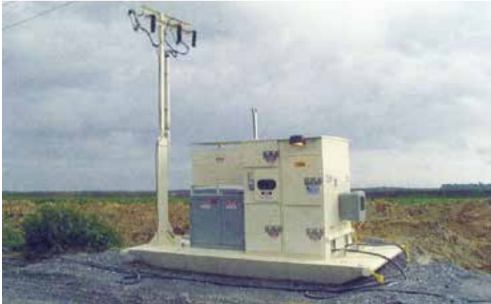
500 kVA Portable Substation with Winch-Operated Fold-Down Tower
