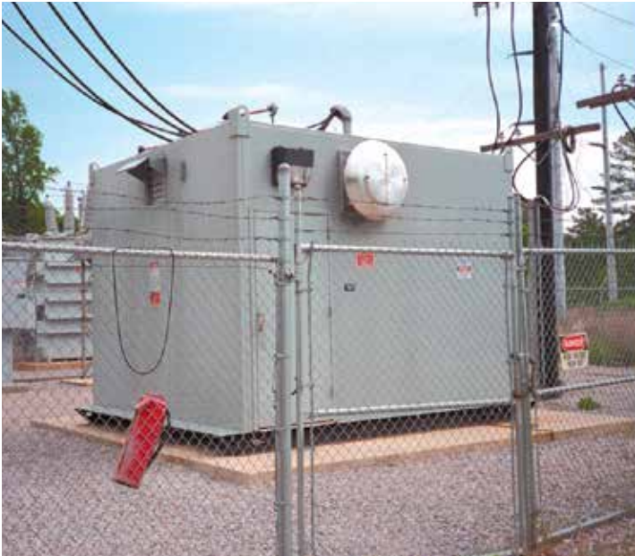
Engineered Substation with bullet-resistant exterior skin for rural location.
