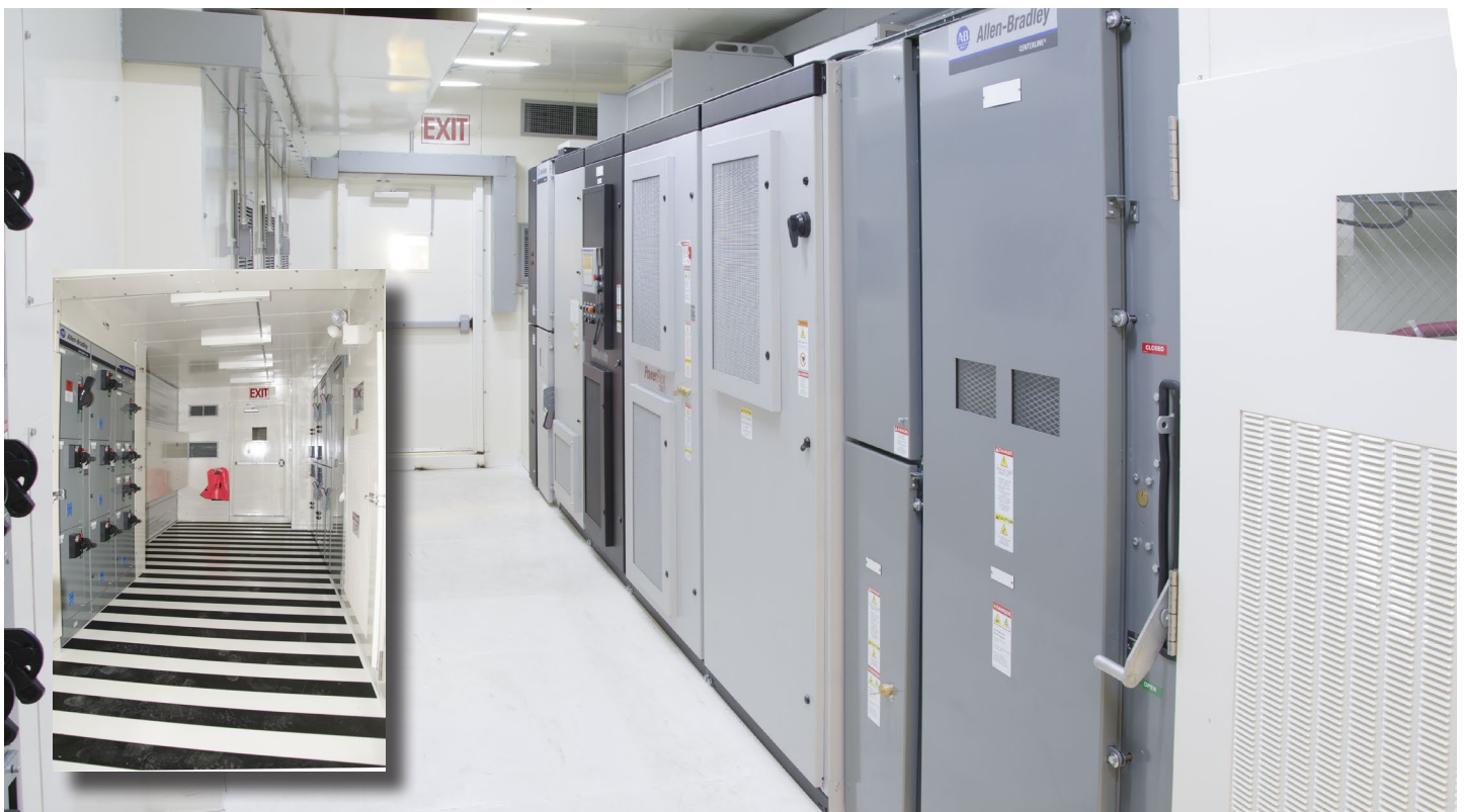
Line Power E-Houses Can Be Equipped With Variable Frequency Drives As Shown Above or With Across-The-Line Full-Voltage Starters As Shown in the Inset
