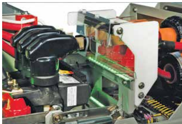
Disengaged and Grounded Contactor (Lit Green)
